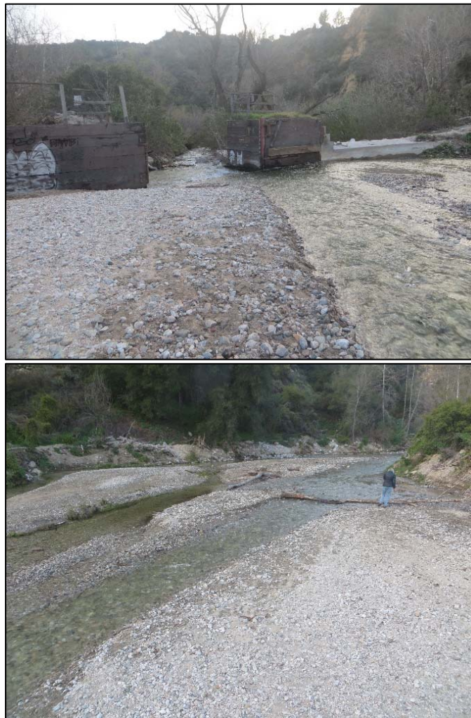
Figure 3-11. Top, the two right-most barriers and the attached weir at the downstream end of the sediment trap. Bottom, view upstream of the sediment deposit.
