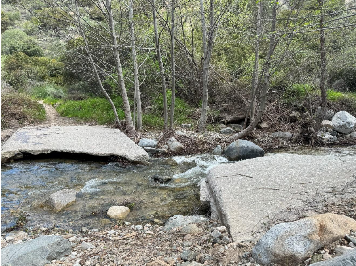
Figure 13. Deteriorated Arizona crossing at river mile 4.85.
