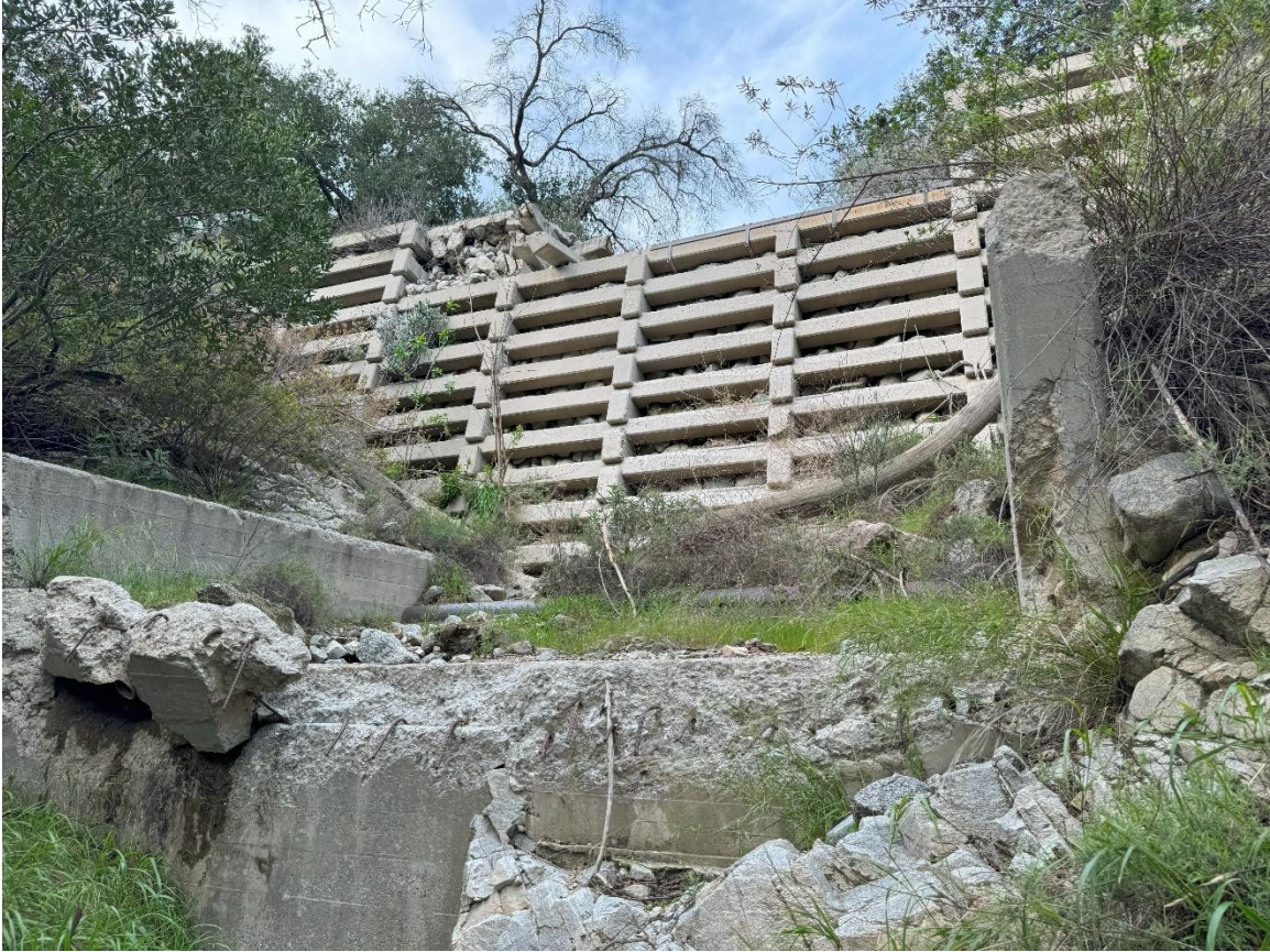
Figure 10. Debris dam on western tributary at river mile 3.43.
